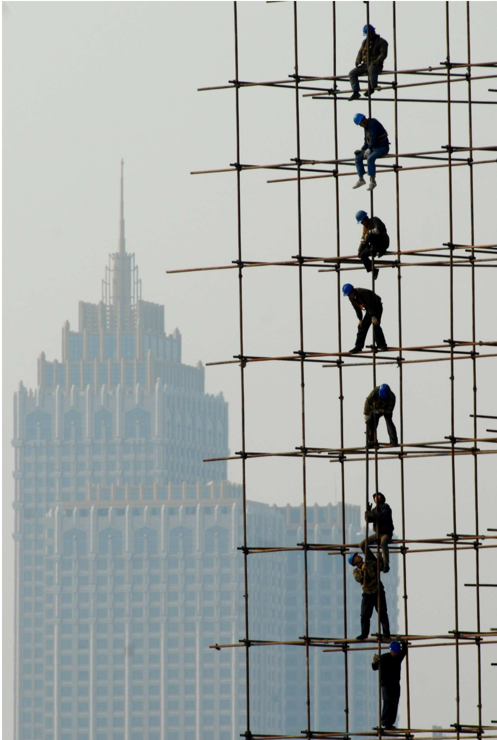
Workers erect scaffolding in Shenyang in NE China (From The Guardian 24 March 2009)
