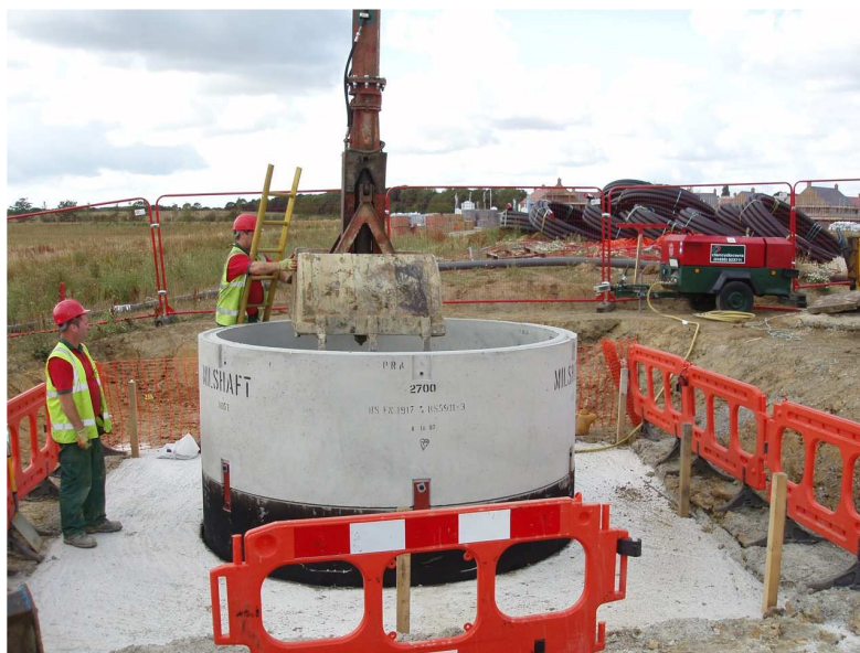
An actual installation, showing bulk excavation using a grab on an excavator
