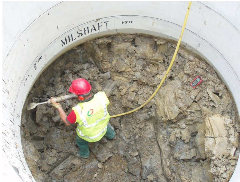
Hand excavation at the cutting shoe, allowing the caisson to sink in a controlled way
